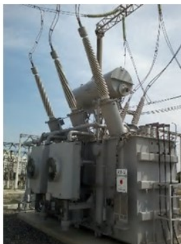
Mushviq substation (grant, 2006)
