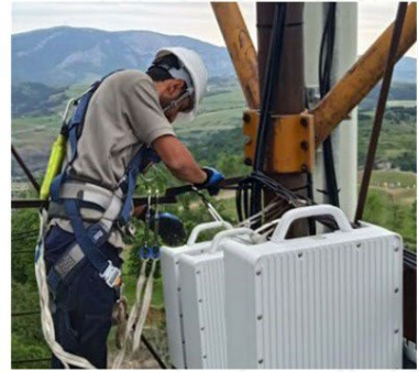
Mobile Base Station
